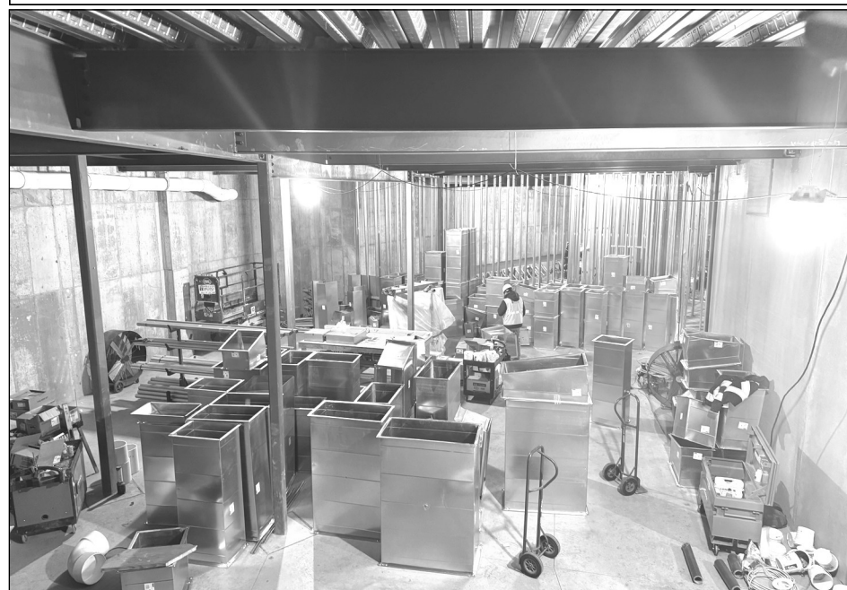
Pictured above is the mechanical room.
