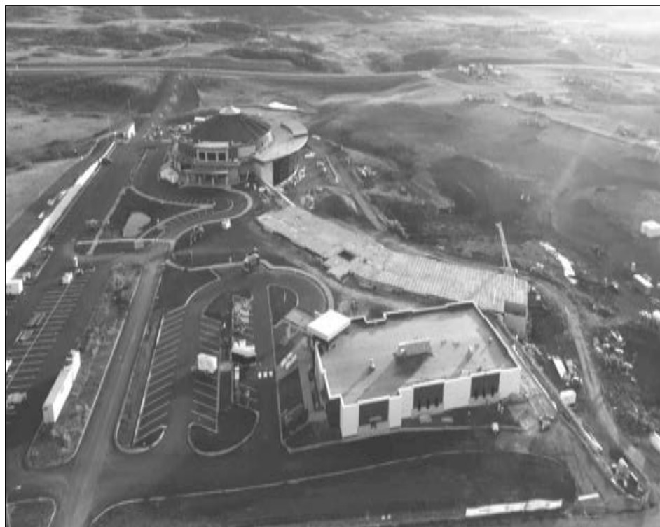
December 2025- Here is a landscape photo of the construction here in Mandaree this picture was taken by Jesus Leyva. This is how the construction looked earlier before the snow came.
