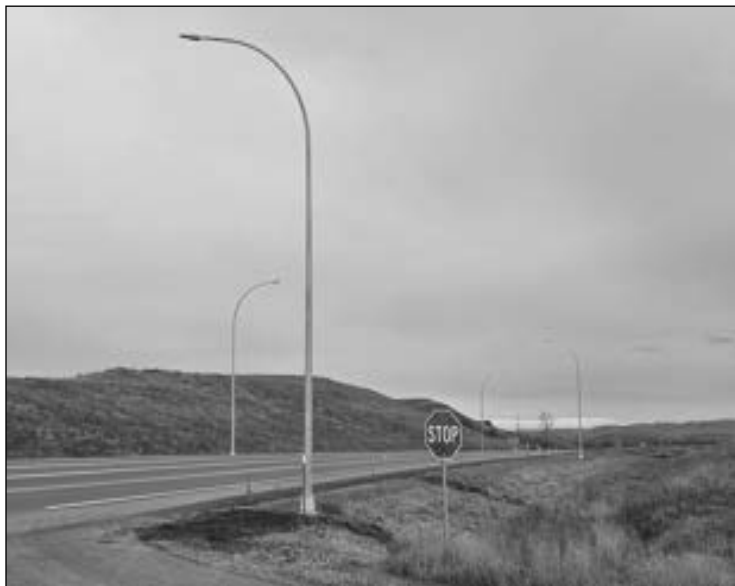
For November 2025-New lights displayed on Highway 22.
