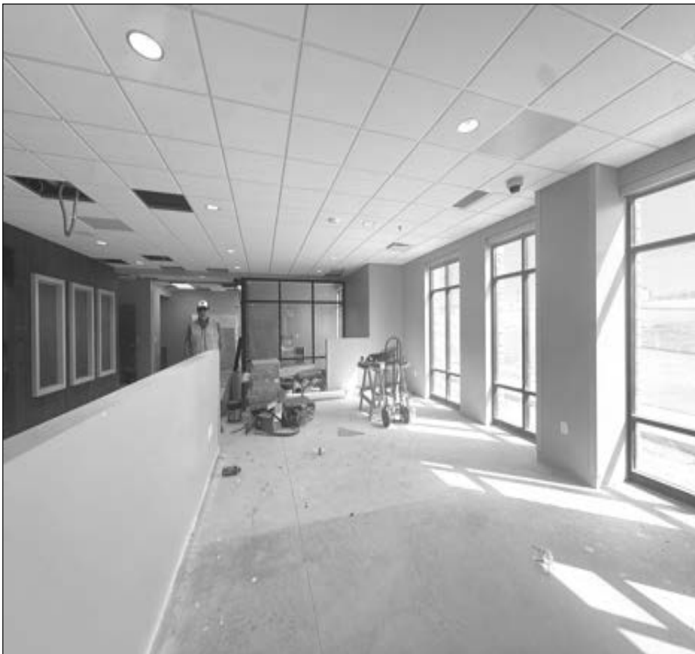
This is where the waiting area will be for patients after they get checked in for appointments. This lobby area is still undergoing construction.
